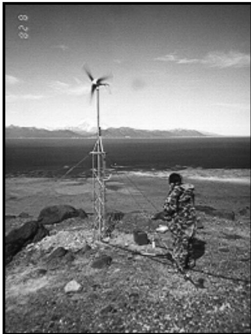
Figure 25: Wind generator installed at station AUP/AUB on Augustine Volcano. Iliamna Volcano is showing in the background.
