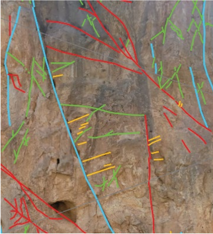
Figure 3.12. Mode I fractures (yellow) perpendicular to bedding surface (blue) indicating outer-arc stretching.
