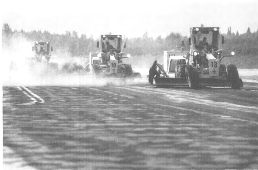
Figure 2. Road graders scrape ash from runways at Anchorage International Airport on August 19, 1992. Road scrapers could effectively move the ash only after it had been sprayed and dampened with water. However, too much water produced a slurry that could not be moved effectively. Dampened ash was scraped into furrows and then scooped up using front-end loaders. Some ash resuspended in the air would settled back onto runways and planes, and thus delayed aircraft cleanup. Photograph by Erik Hill courtesy of Anchorage Daily News.
